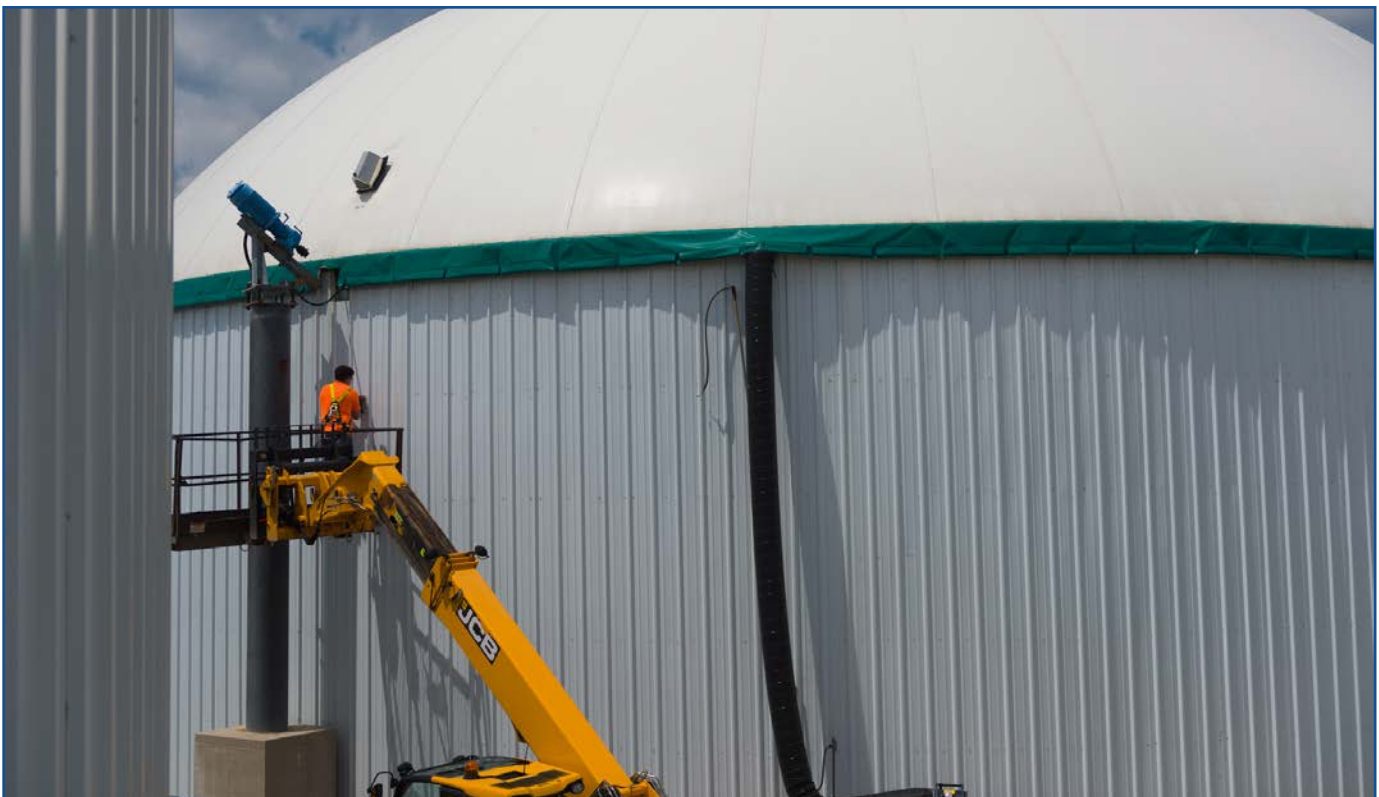
Photo 7: Dairy Biogas Anaerobic Digester Facility, Clean Fuel Partners, LLC, Dane, WI
