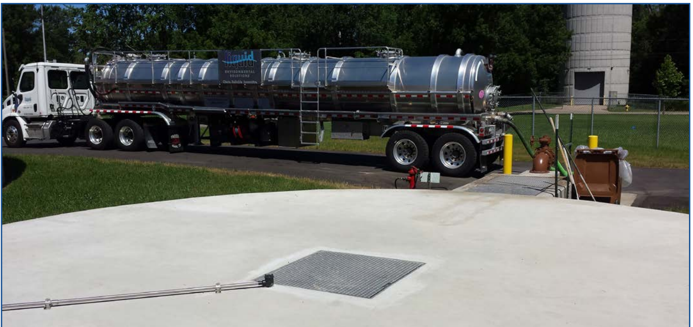
Photo 3: High strength equalization tank with truck, Waste Water Treatment Facility, Stevens Point, WI
