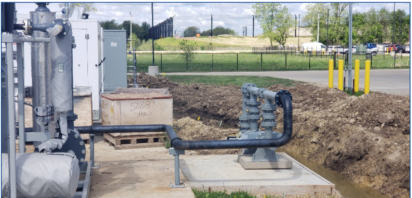
Photo 5: Pipeline injection of biogas from a Dane County Landfill, Dane County Public Works, Madison, WI
