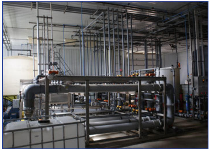
Aqua Innovations reverse osmosis system
