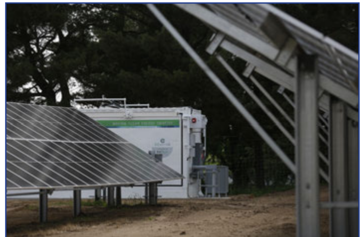
Battery storage with solar arrays
