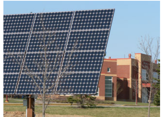
Photo CP3: In 2007, a 3.7 kW photovoltaic dual-axis tracker system was installed at River Falls High School. A kiosk and website provide real-time energy production data. The system provides an estimated 5,236 kWh of energy per year. (Photo courtesy of River Falls Municipal Utilities)
