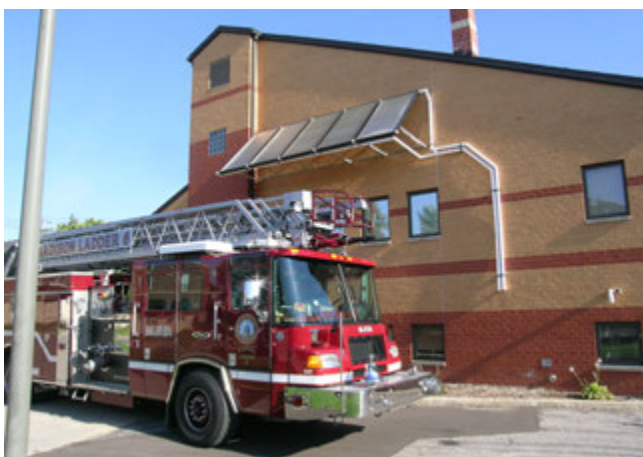
Photo CP4: Solar hot water heaters were installed at Fire Station 6. (Photo courtesy of the city of Madison)
