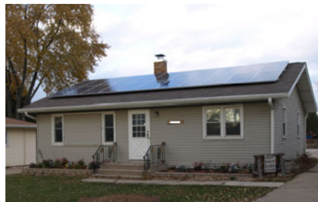
Photo CP5: A solar installation in the city of Madison. (Photo courtesy of the city of Madison)
