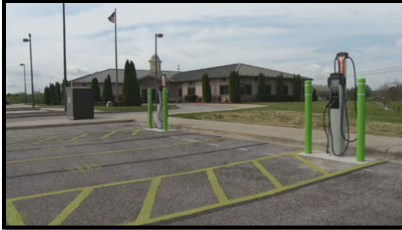
Lake Mills two vehicle charging location outside of city hall.
