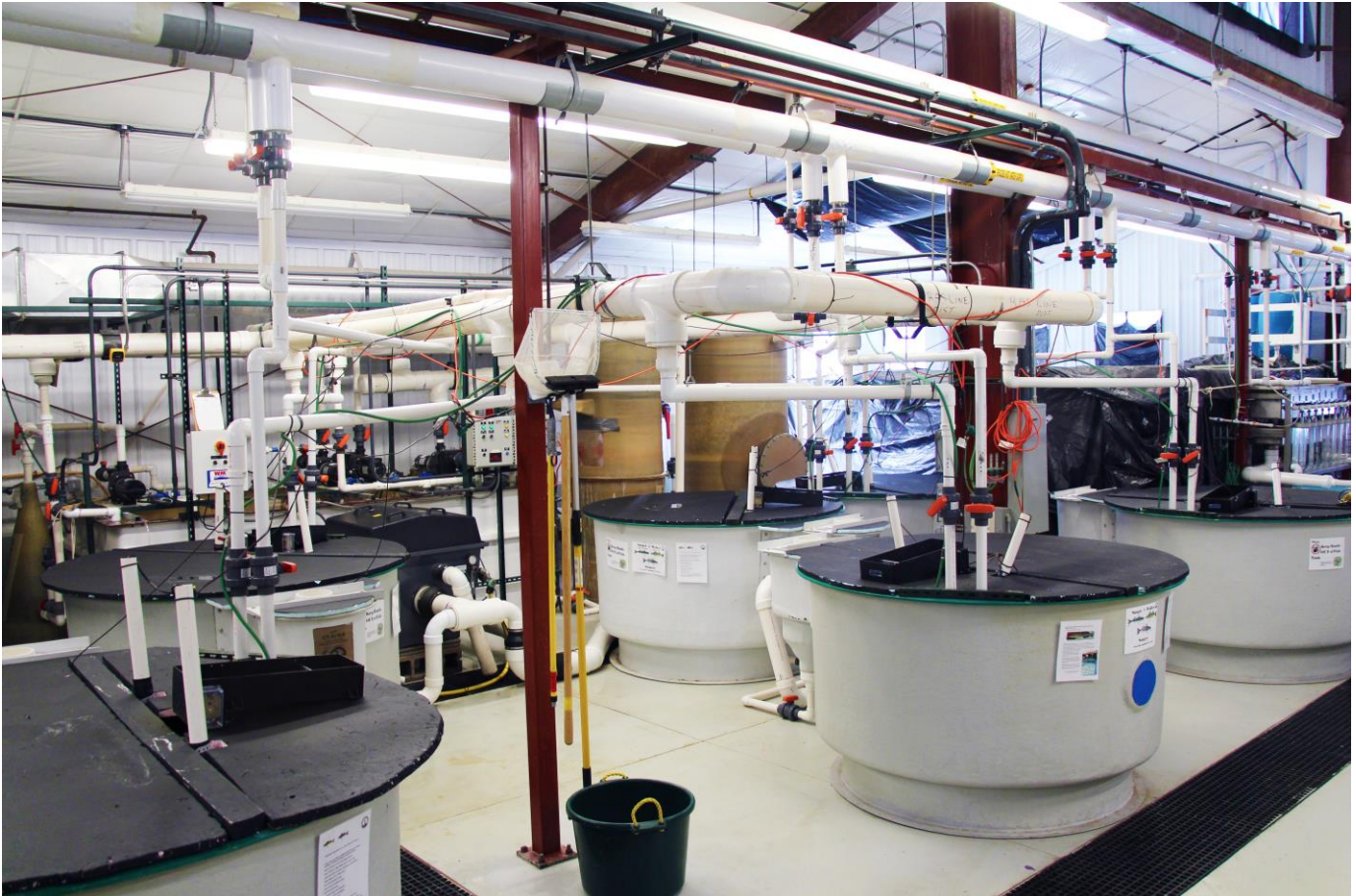
Fig. 48. A water recycle system at UWSP-NADF. The system above consists of six (6) 2.32 m 3 “Cornell-type” culture tanks with attached radial flow settlers, a micro screen drum filter, a 8.0 m 3 sump with overflow and float valve controlled freshwater inflow, biofilter pump station, sand cyclonic biofilter, carbon dioxide stripping column w/fan, distribution pump station, ultra violet treatment unit, oxygen cone, overhead distribution pvc piping, and paddle wheel flowmeter.
