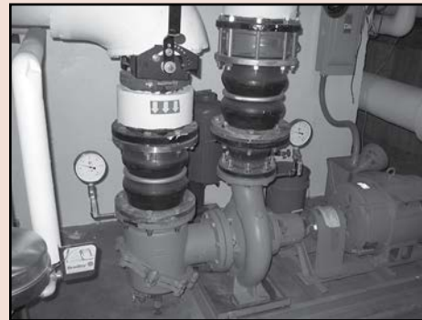
This pump circulates hot water from the boiler room to various parts of the school building.
