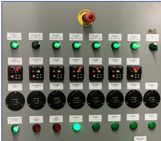
Digester heat pump monitoring
