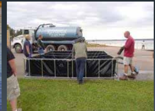
Removal of Treated Water
