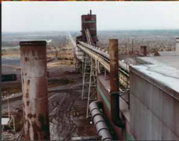
Processing plant to rail loadout
