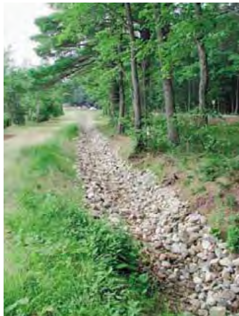
A swale constructed along this roadway captures road runoff and prevents it from entering the lake, which is to the left.
