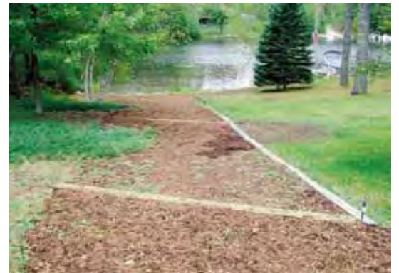
Waterbars along the path slow flow and divert runoff into the vegetated area.
