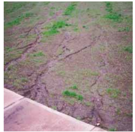
Shallow rills forming from the concrete sidewalk runoff.
