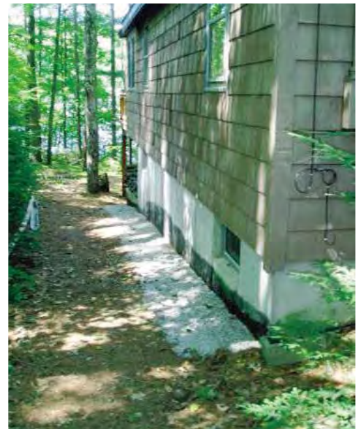
An infiltration trench was constructed to catch roof runoff at this lakeside home.
