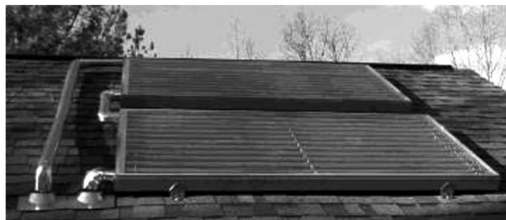
Solar panels collect thermal energy from the sun to heat water for household use. Picture from North Carolina Sustainable Energy Association.
