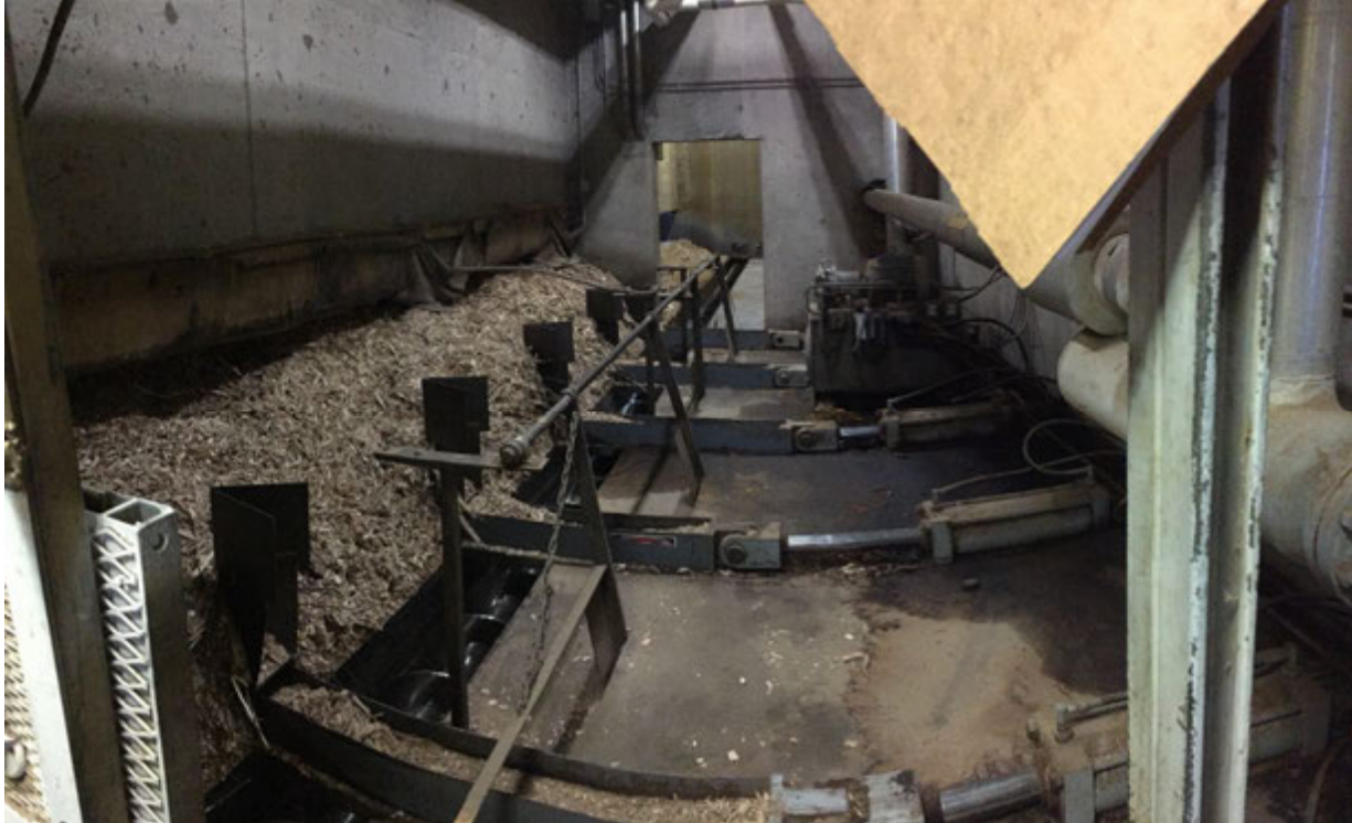
Photo 1: Wood Chip Auger Delivery System For Barron School District's Wood Boiler Heating System, Barron, WI.
