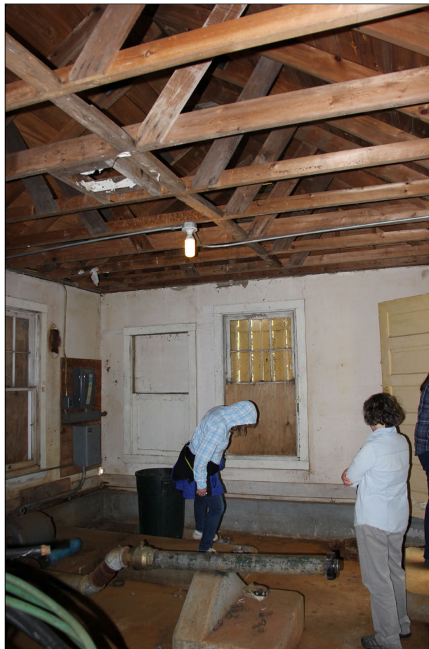
Figure 109. —Interior of the Hugo Sauer Nursery pumphouse #2 (map area #14) facing north, 2019.
