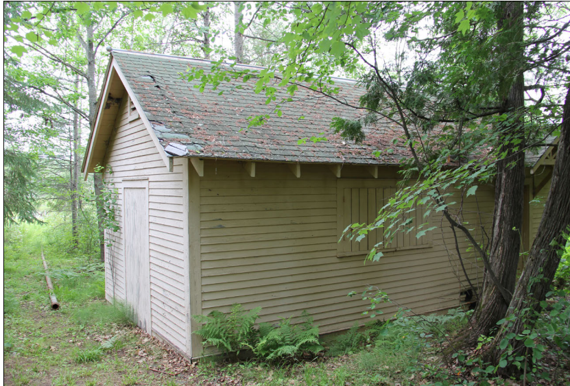
Figure 106. —Hugo Sauer Nursery pumphouse #2 (map area #14) facing northwest, 2019. The pipe on the ground to the left leads towards an inlet of Langley Lake where water was pumped from.
