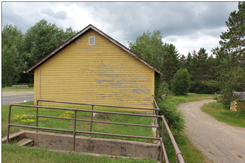
Figure 85. —Hugo Sauer Nursery seed storage shed (map area #6) facing west, showing the adjacent steps through the retaining wall, 2019.
