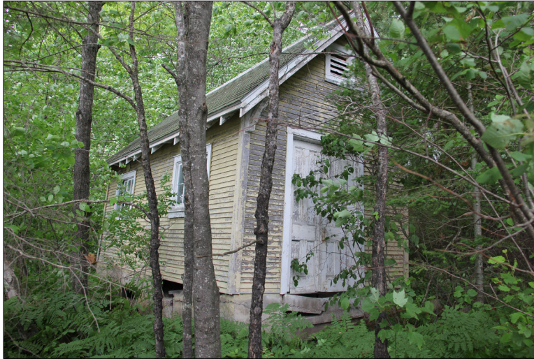
Figure 91. —Hugo Sauer Nursery pumphouse #1 (map area #8) facing northeast, 2019.
