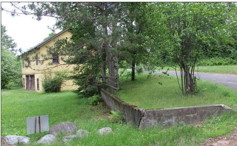
Figure 126. —The start of the 400-foot-long concrete retaining wall behind warehouse #1 (map area #5), 2019.
