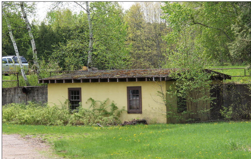
Figure 79. —Remaining lower floor of the Hugo Sauer Nursery seed extractory (map area #4) facing south, 2019.
