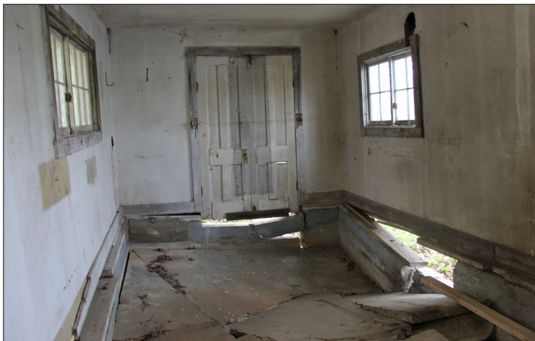
Figure 93. —Interior of the Hugo Sauer Nursery pumphouse #1 (map area #8) facing south, 2019. Note the deteriorating foundation.
