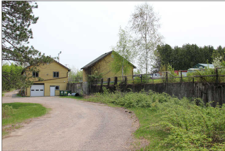
Figure 127. —Segment of the 400-foot-long concrete retaining wall behind the seed storage shed (map area #6) and ending at cone shed #2/ packing plant (map area #7), 2019.
