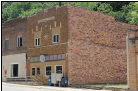
A blank brick wall on the side of the Linn Grove Post Office would be ideal for a mural.
