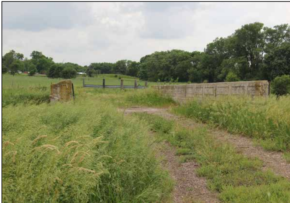
Brooke Creek Bridge, built in 1909, crosses a tributary of the Little Sioux River south of County C16, the southern stretch of the byway loop.
